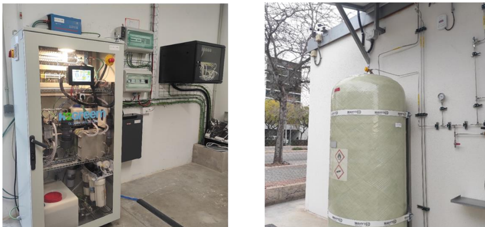
Figure 4. Prototype for solar energy production, storage and management.
